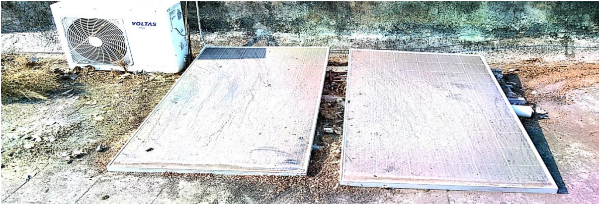
2 KVA Solar Power Generation Unit in IQAC Office (Office Building)
